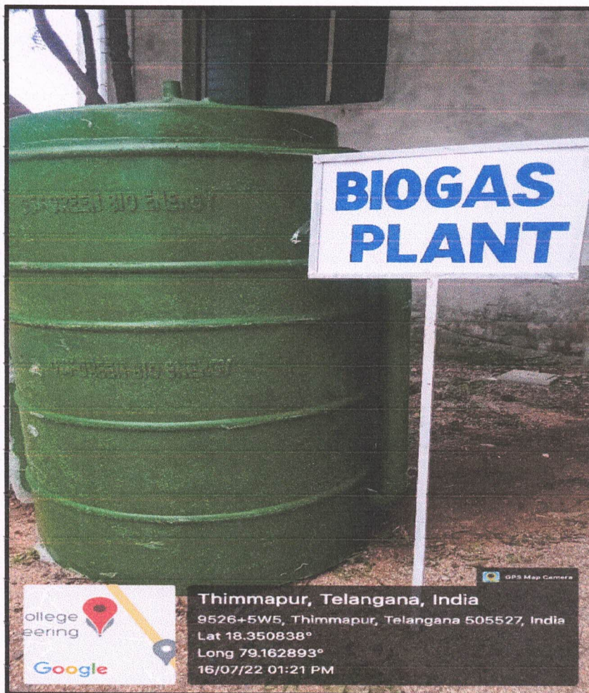
Biogas plant at VGSE
